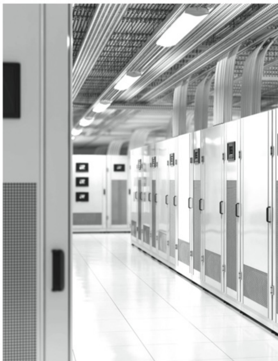
interior of Volta Data Centre
